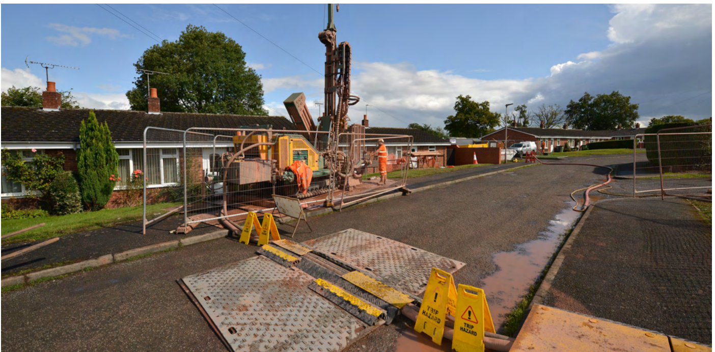
Boreholes being drilled for a shared ground loop heat pump scheme. Courtesy Kensa Heat Pumps.
