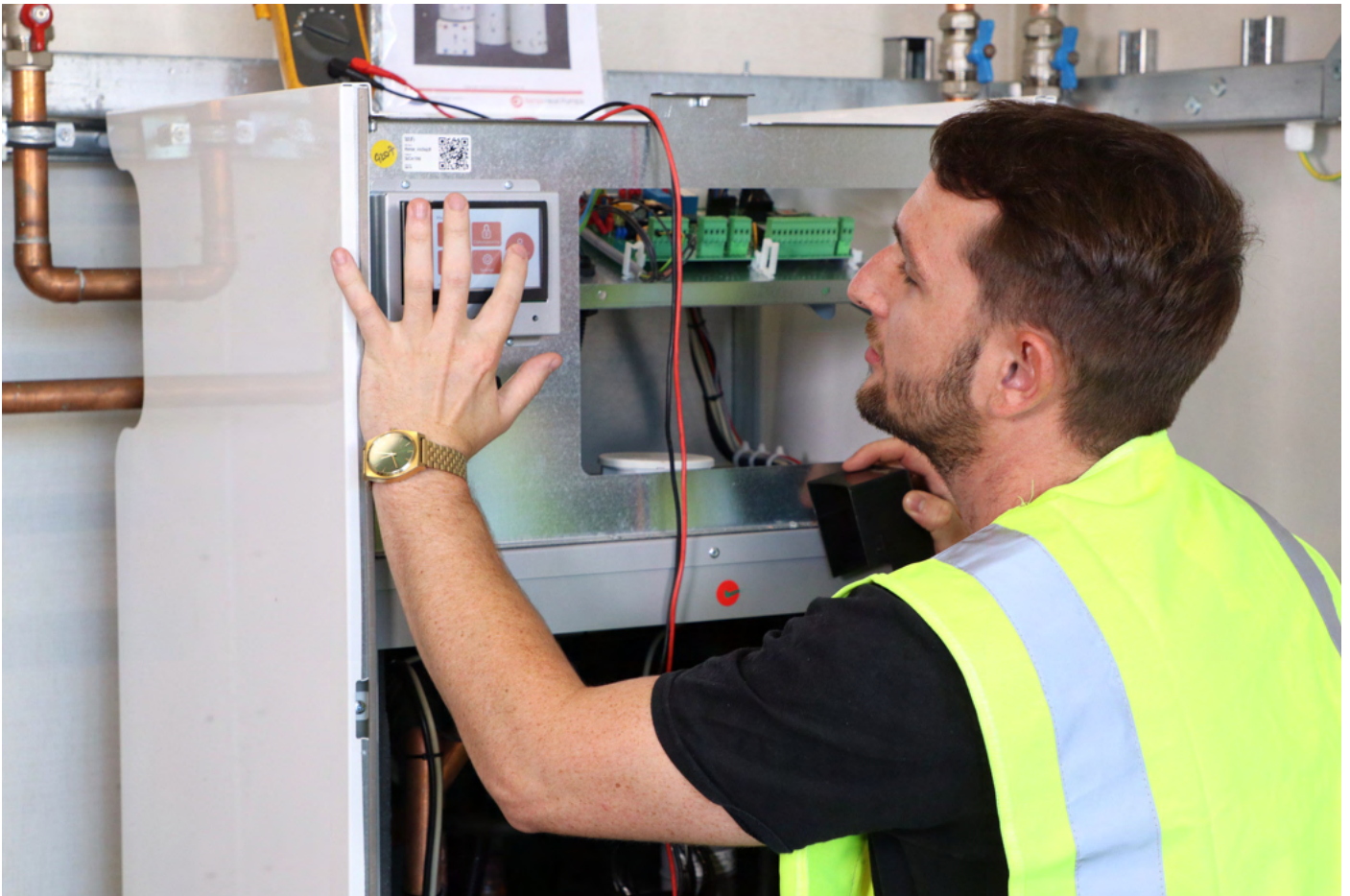
A ground source heat pump being installed. Courtesy of Kensa Heat Pumps.
