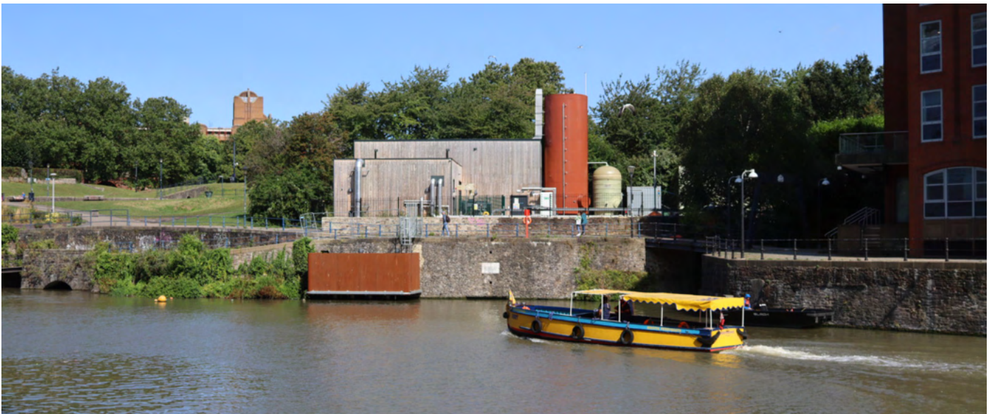
Bristol Castle Park Energy Centre Water Source Heat Pump. Courtesy Star Renewables.
