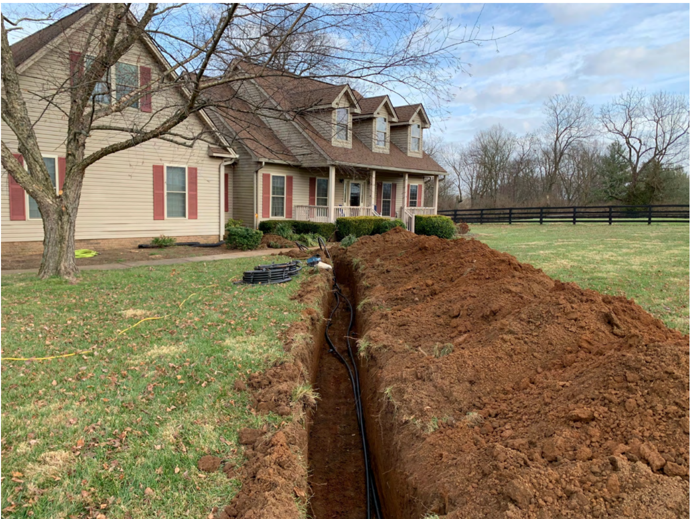
A trench for a ground source heat pump ground array. Courtesy of Danielsen_Photography/Shutterstock.
