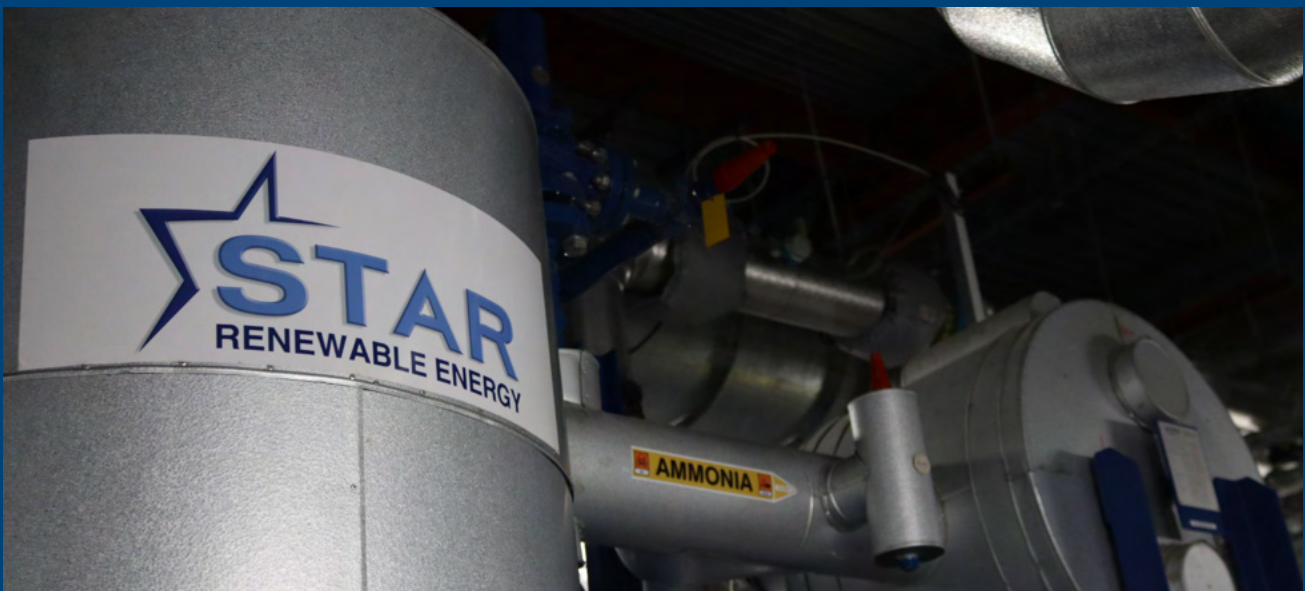
Internal image of Bristol Castle Park heat pump. Image courtesy of Star Renewables.
